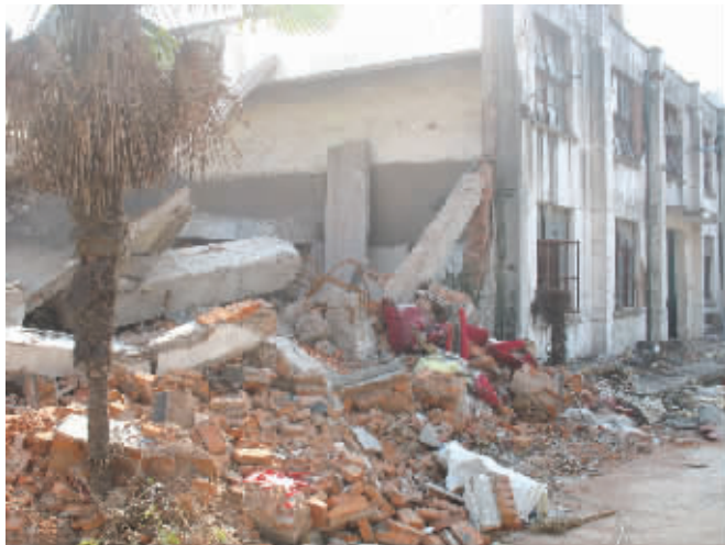
倒塌的厂房里到处都是碎砖
