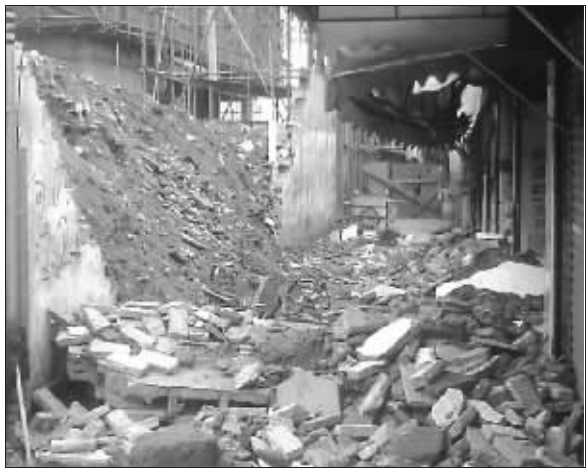
墙体坍塌后,弄堂堵了起来
