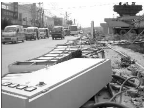
地铁施工围挡被推倒
